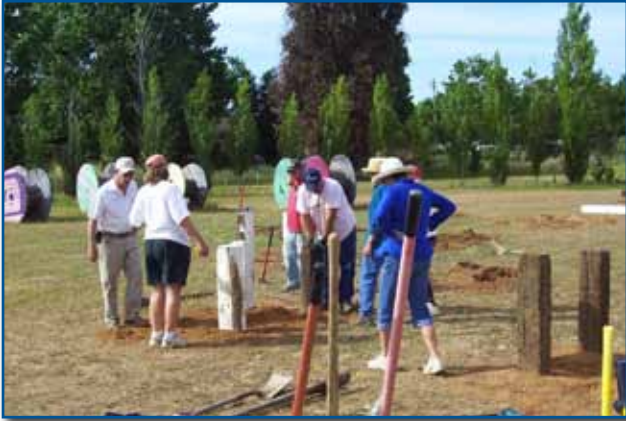
Volunteers hard at work, setting the railroad tie sides of the buildings
